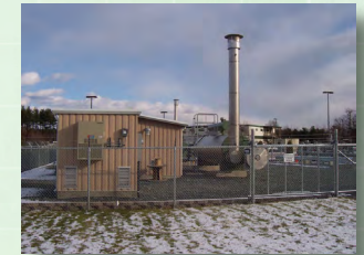
Metering and Regulating Station
